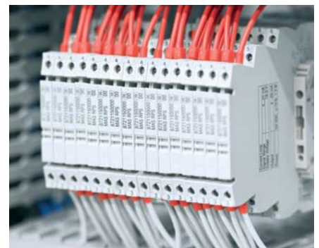
MICROANALOG analogue signal converter with electrical isolation. Easy to set using a DIP switch.
